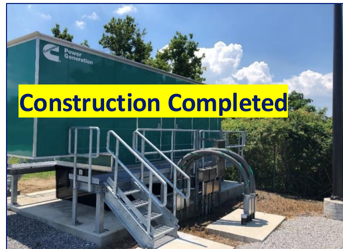
Lake Timberlane New Lift Station & Generator ($2.6 Million)
